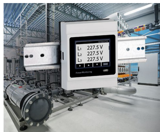
Monitoring of electrical variables
